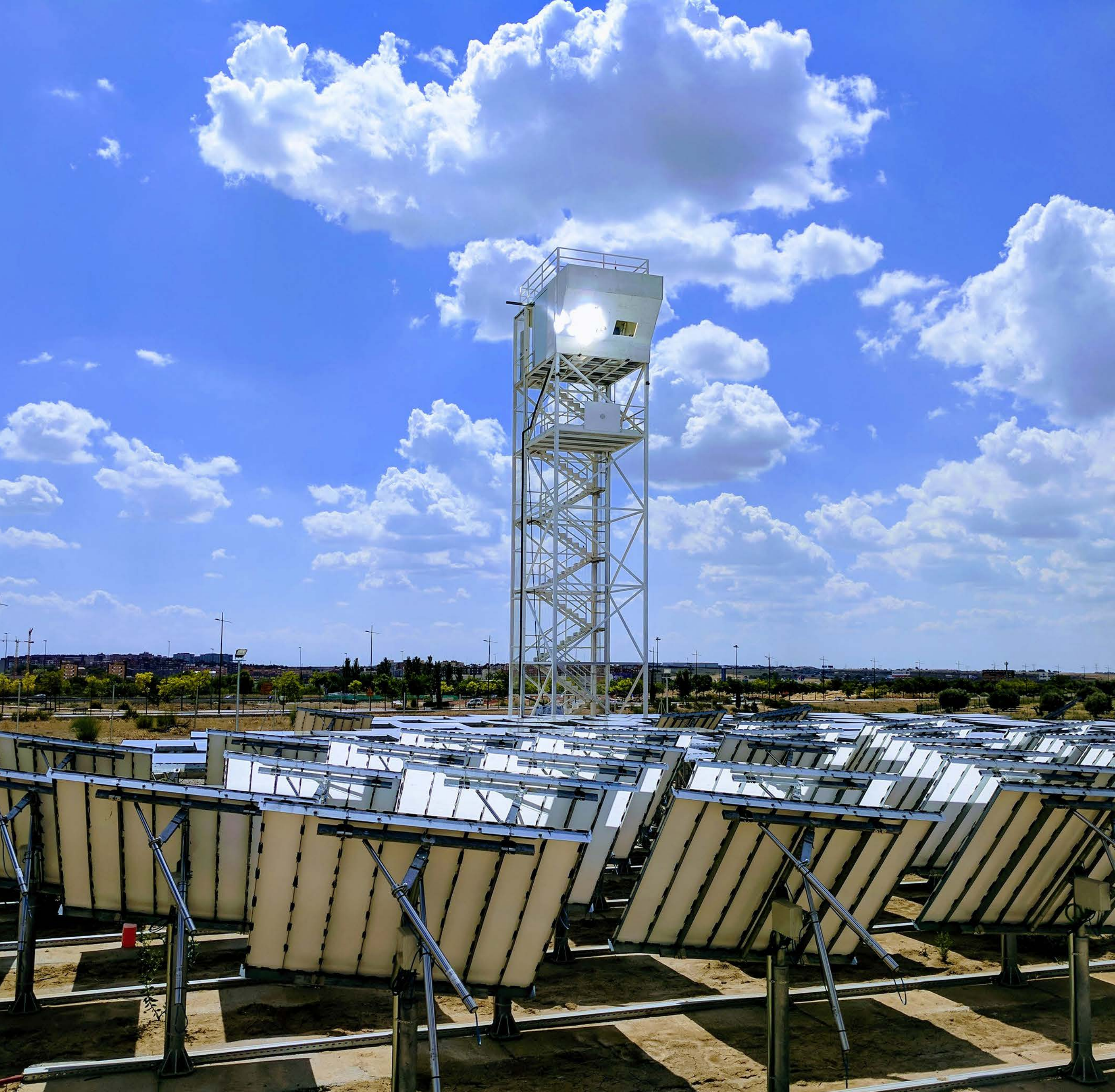
Fig. 3: Photograph of the solar tower fuel plant located at IMDEA-Energy, Madrid. A field of sun-tracking heliostats focuses the direct solar irradiation onto the solar reactor positioned at the top of the tower. The solar reactor co-splits \text{CO}_2 and \text{H}_2\text{O} via the ceria-based thermochemical redox cycle and produces a desired mixture of \text{CO} and \text{H}_2 (syngas), which is finally processed via Fischer-Tropsch synthesis to kerosene [4].
