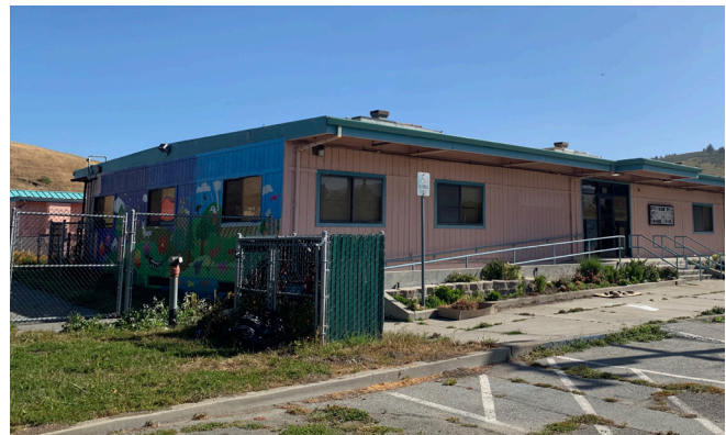
LHPUSD recently completed an assessment of their facilities and the projected cost of deferred maintenance.
